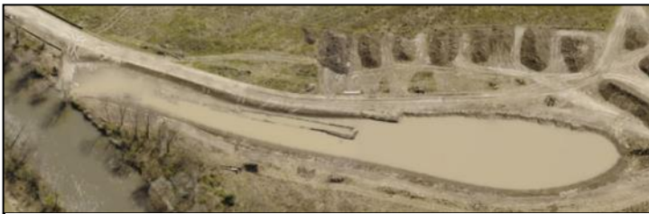
2.5-acre backwater spawning area under construction. Two very similar features are also in-progress.
