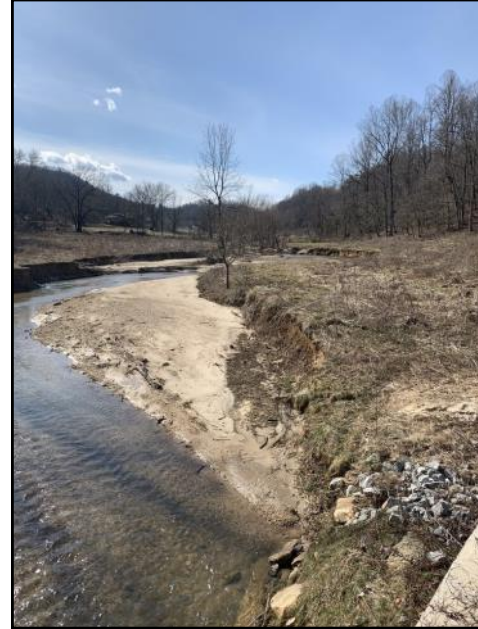
Prior to construction Reedy Patch Creek's streambanks showed critical erosion due to limited stabilizing vegetation.
