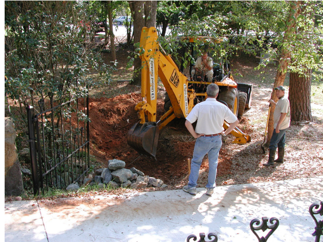
Figure 6-6. Communicating with a contractor during the construction of a bioretention area / rain garden
