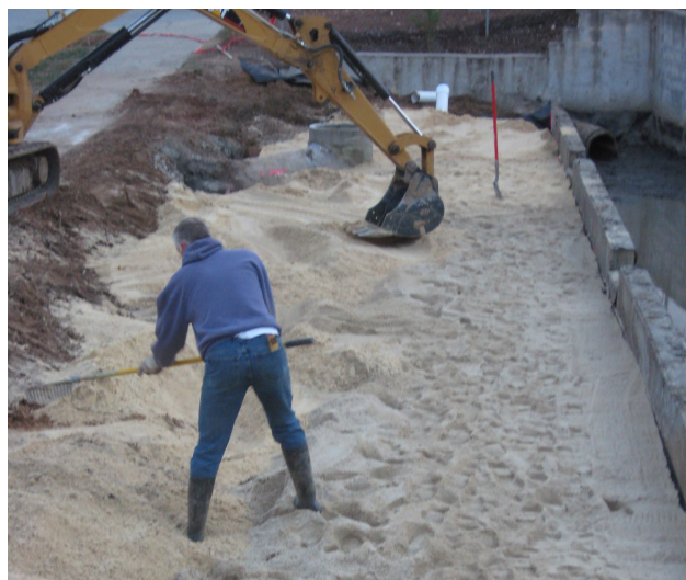
Figure 4-14a & b. Sand filter under construction A drainage pipe underlies a sand-filtering media. Most sand filters do not allow for infiltration.
