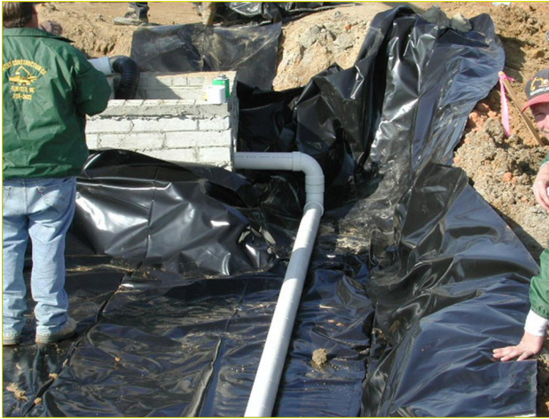
Figure 4-15a & b. An upturned underdrain creates a sump in the bottom of the bioretention cell (top); outflow from an upturned underdrain (bottom)
