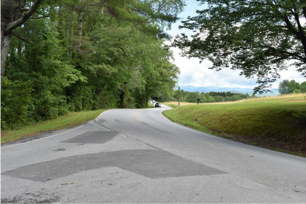
Project beginning, SR 1533 (Everett Road), intersection with SR 1534 (Hart Road), view to west
