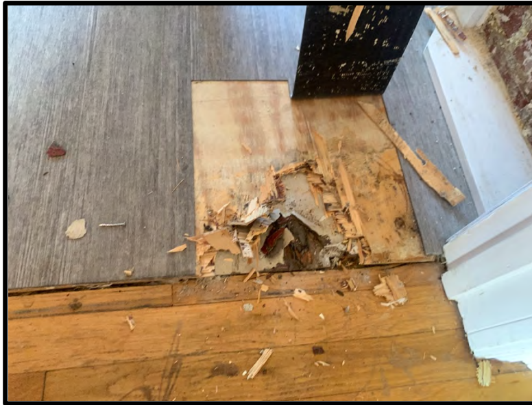
Photo No. 1 – Homogeneous A-07 Brown Wood Square Pattern Vinyl Sheet Flooring with underlayer of Red Vinyl Sheet Flooring and Black Mastic (Only Underlayer of VSF and Mastic is Asbestos Containing)
