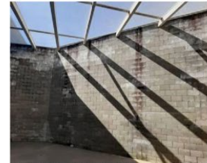
Figure 11 – Mold and efflorescence at minimum housing recreation yard
