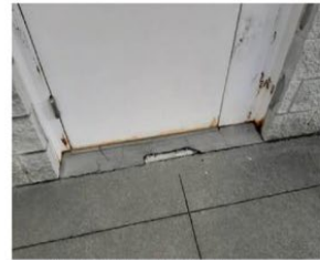
Figure 7– Rust at exterior doors and frames.
