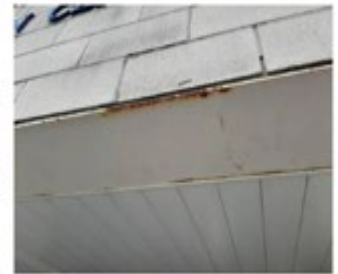
Figure 2 - Example of rust at intel
