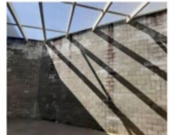
Figure 11 - Mold and efflorescence at minimum housing recreation yard
