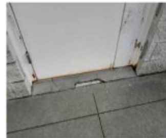
Figure 7 - Rust on exterior doors and frames.
