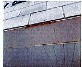
Figure 2 - Example of rust at inlet
