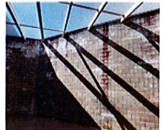
Figure 4 - Mold and efflorescence at minimum housing restriction yard
