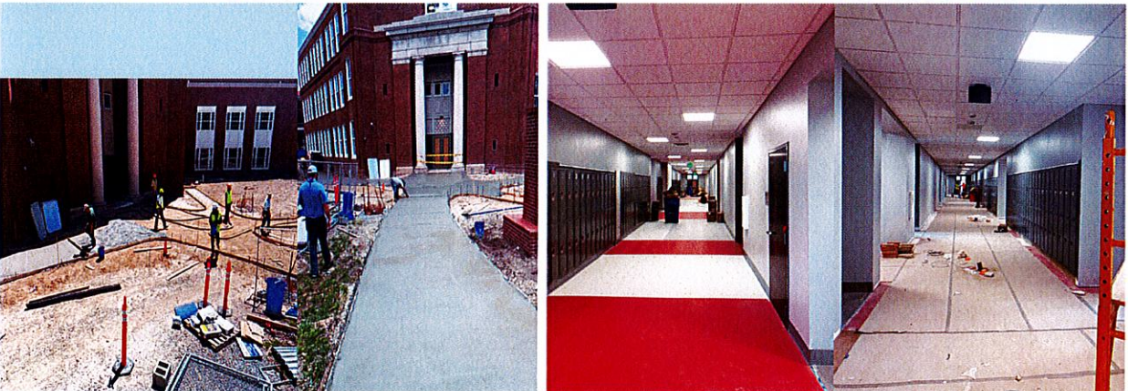
Paving projects continue at Hendersonville and Etowah Elementary, Apple Valley Middle, and North and
