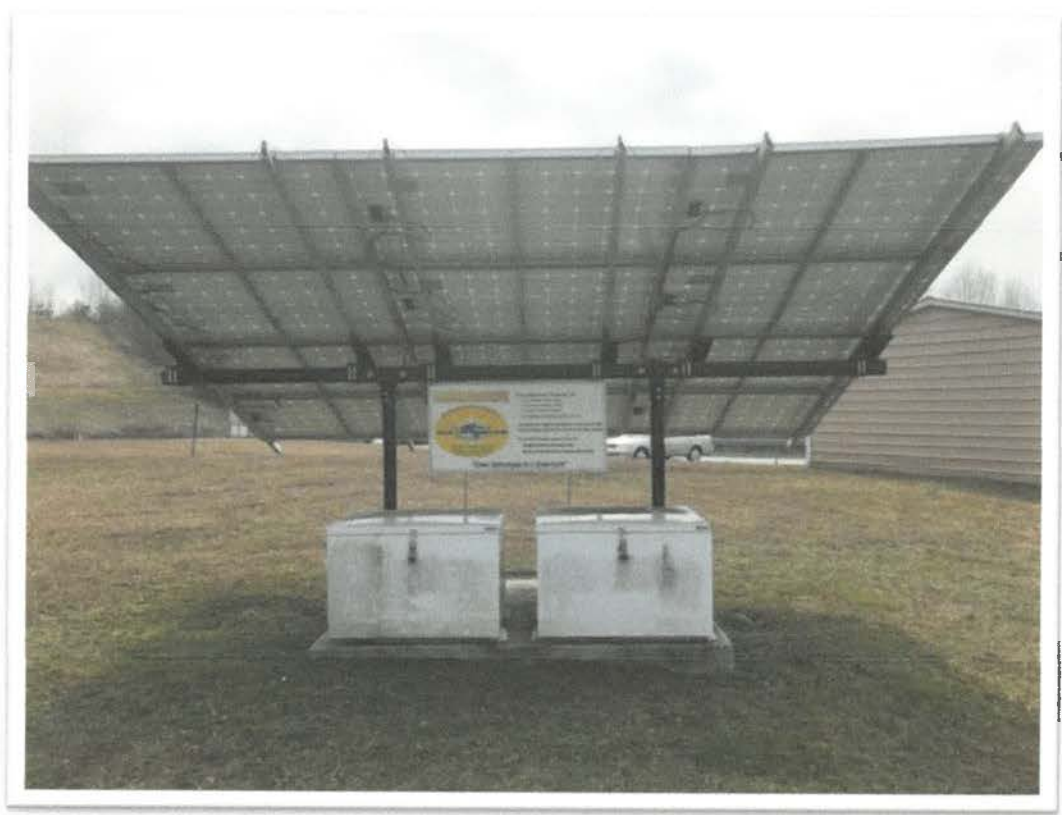
Figure 4: Solar Panel Battery Bank
