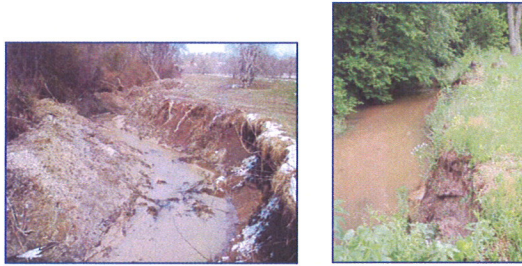
Severe Erosion on Devils Fork Bank
