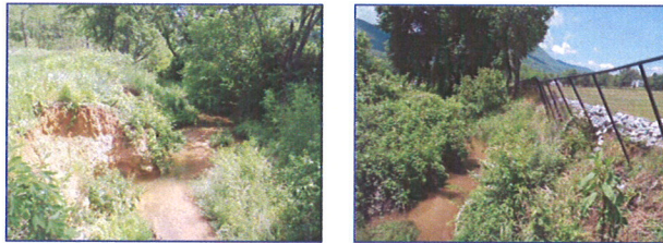
Severe Bank Erosion on Mud Creek
