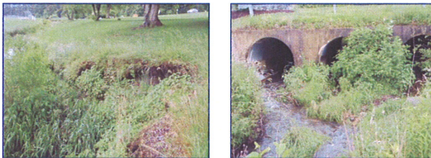
Erosion on Mill Pond Creek Bank
